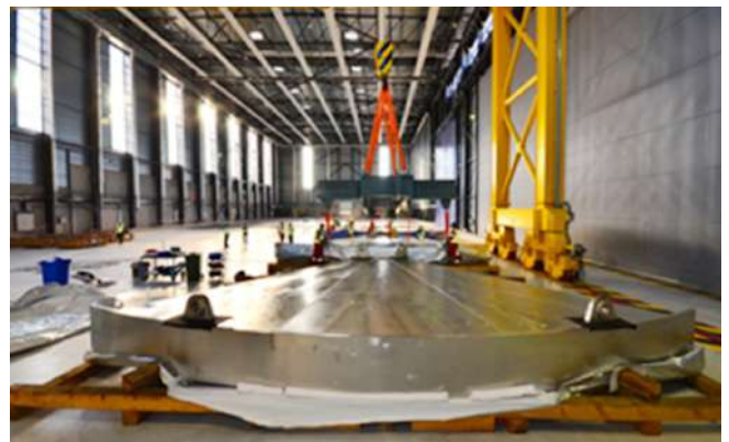
Figure B.2.4 Cryostat – Base Tier 1 components delivered at Cryostat workshop on ITER site
