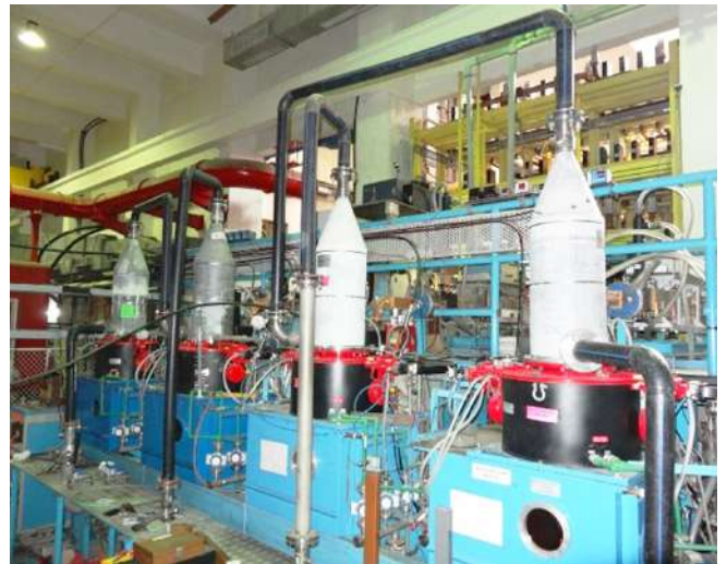
Figure A.1.2.3.3 A photograph showing all the four klystrons
