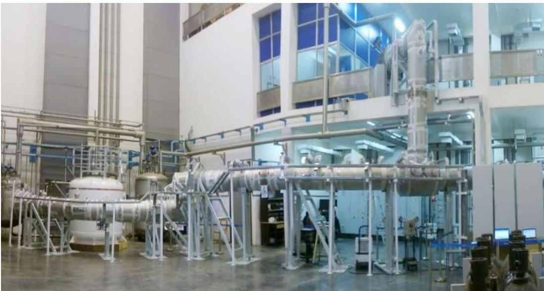
Figure B.2.7 As installed Pre-series Cryo-Line PTCL-1) in ITER-India lab
