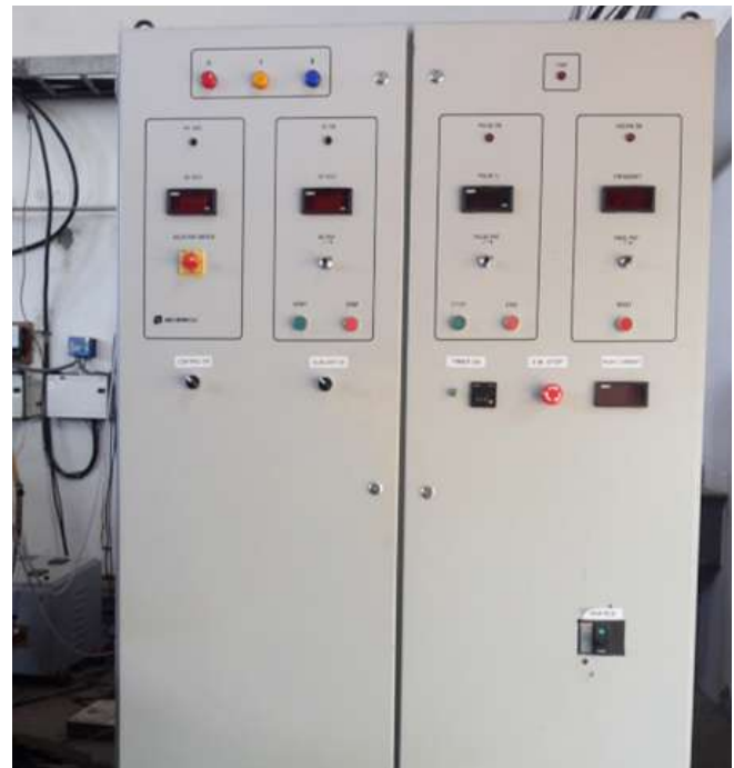
Figure B.1.5 Image of the 25KW pulsed power source
